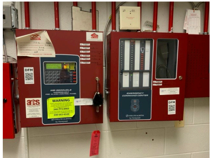
28 - FIRE ALARM PANEL
