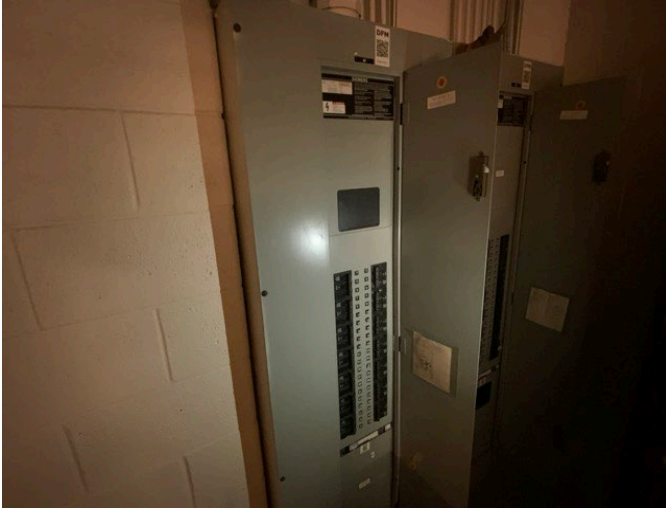
25 - TYPICAL DISTRIBUTION PANEL
