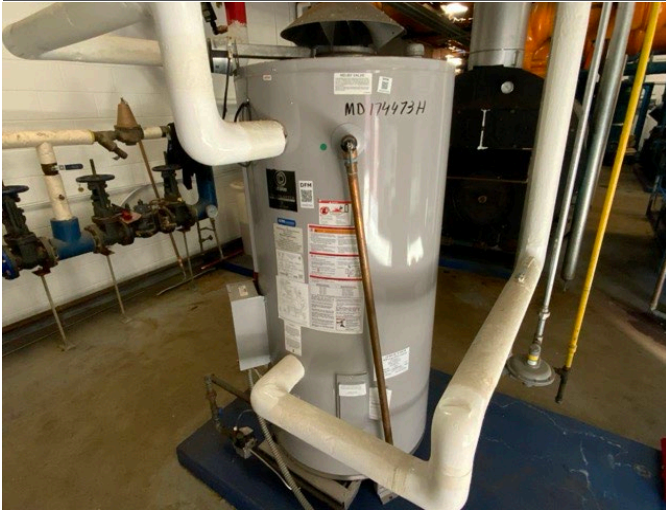
13 - GAS WATER HEATER
