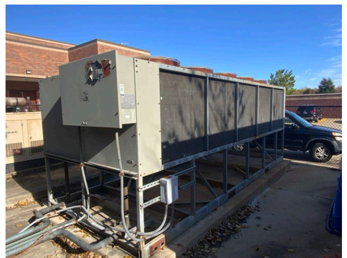
18 - AIR COOLED CHILLER
