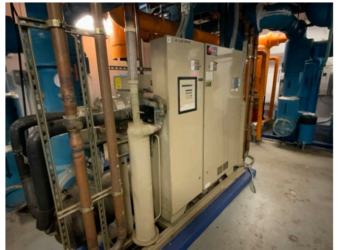
16 - WATER COOLED CHILLER
