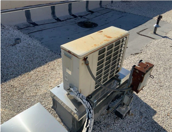
19 - DUCTLESS SPLIT SYSTEM
