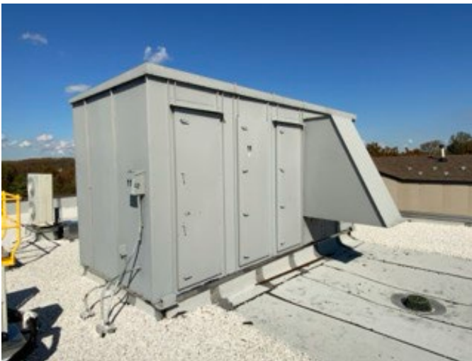
21 - TYPICAL EXTERIOR AIR HANDLER
